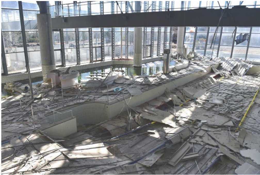
A pool whose roof has fallen in is seen at the "Rifure Tomioka" hot spring facility in Tomioka, Fukushima Prefecture, on March 2, 2018, nearly seven years after the quake and tsunami disaster. (Mainichi)
