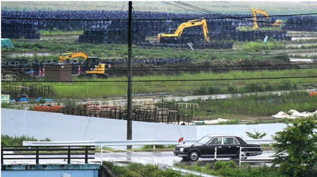
A car carrying Emperor Akihito and Empress Michiko runs on National Road No. 6 in Minami-Soma, Fukushima Prefecture, on June 10. Bags containing radioactive soil are piled up along the road. (Hiroyuki Yamamoto)
